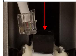
Load Cell Cable Not Connected
